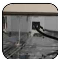
Interior Electrical Outlet
