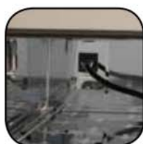
Interior Electrical Outlet
